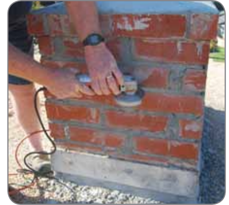
Repointing deteriorated mortar joints is one of the most effective and permanent ways of decreasing water entry into brickwork.
